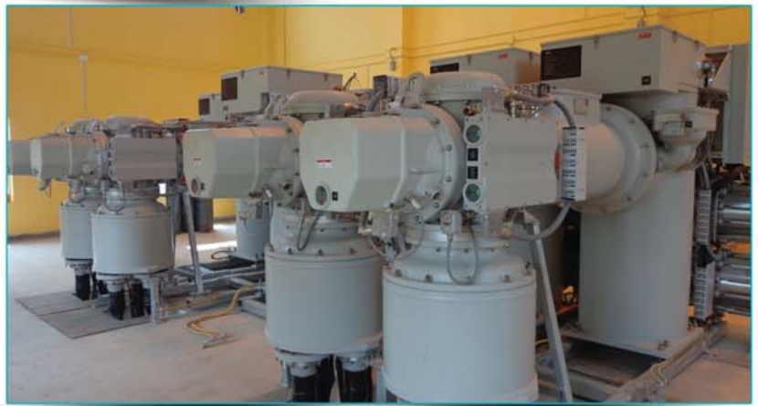
Kuli GI Sub-station
