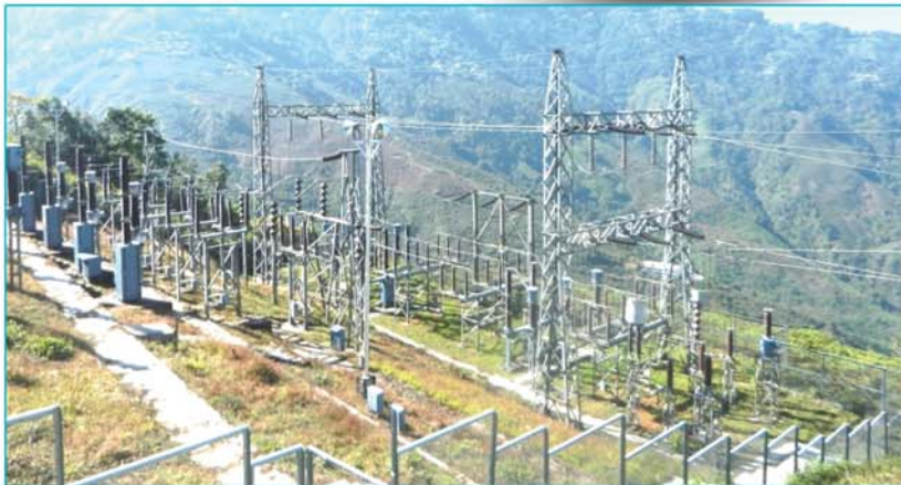
Darjeeling (Lebong) 132 kV Sub-station
