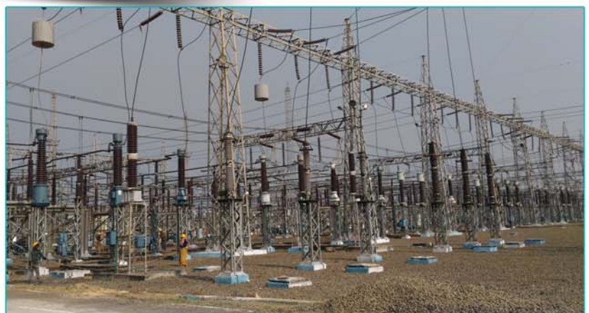
Jeerat 400 kV Sub-station Switchyard
