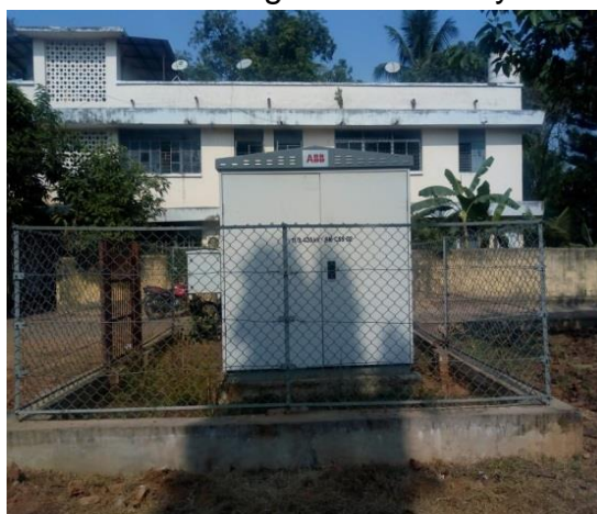
Compact Substation with DT
