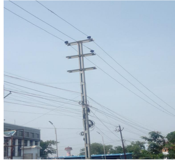
H-Type GI Poles for 11kV and 33kV Lines
