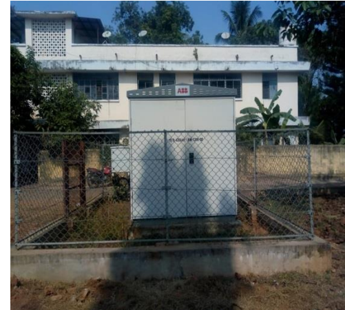
Compact Substation with DT
