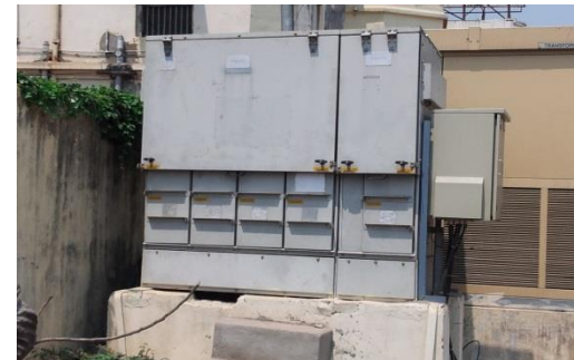
11kV Ring Main Units
