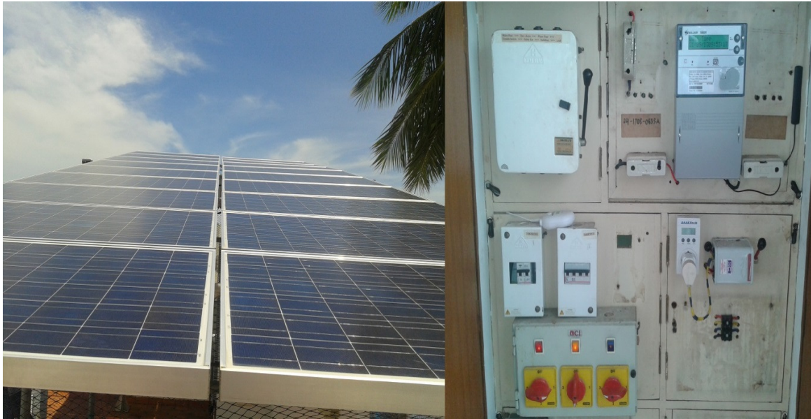
Figure 4: Solar PV modules and Smart meter at consumer – 1 Residence
