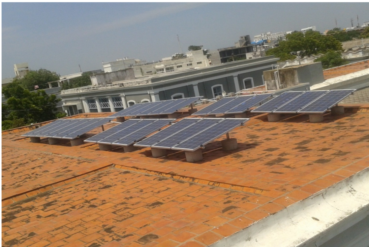
Figure 7: Solar PV module at SAICE
