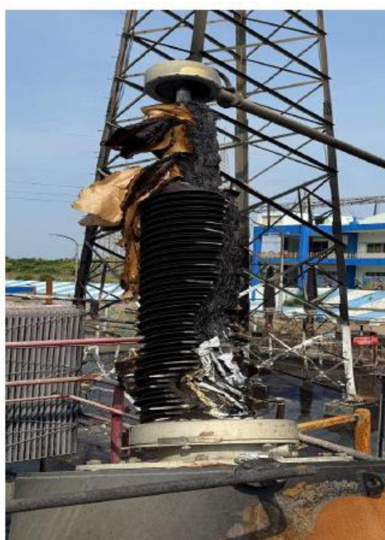
GT HV bushing got damaged
