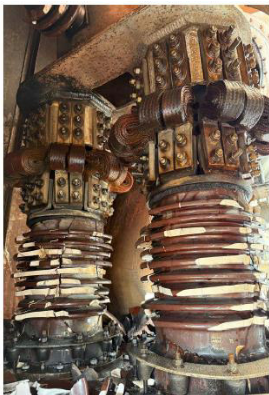
GT LV winding lead terminal insulator damaged
