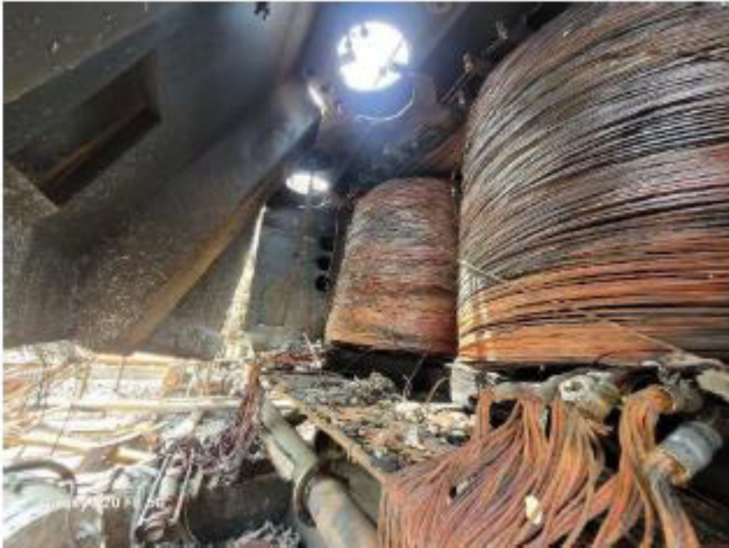
IV side winding (completely burnt)
